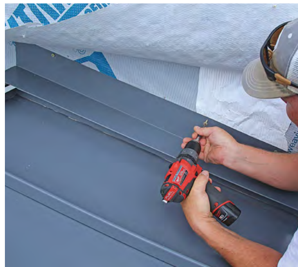
Sidewall flashing. With the Z-strip fastened, sidewall flashing is hooked onto the top of the Z before being fastened to the sidewall through its vertical leg, which will later be covered by the WRB and siding.
