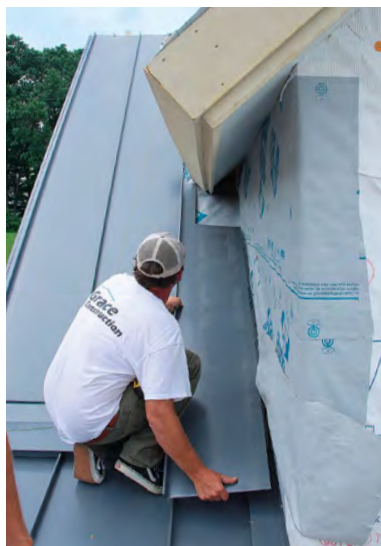
Cut to width. Panels abutting dormers or penetrations are first cut to length and width and then clipped to the neighboring panel.
