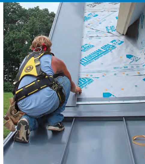
On up the roof. With the transition flashing in place, the same joggle cleats used for valleys are taped and screwed on top to receive the bent edges of the upper roof panels.
