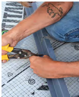
Closed off. Ridge caps and slope transitions use notched Z-strips fit over panel ribs to prevent rain and animals from getting underneath.
