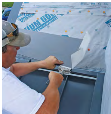
Trim for transitions. With the Z-strip and neoprene closure in place, a slope transition is hooked onto the top leg of the Z. Ridge caps connect similarly.
