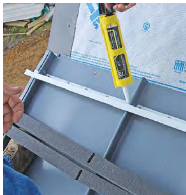
Sealed slope change. After the Z-strip is seated in tape and fastened, it's coated with adhesive and backed up with weatherproofing neoprene strips.
