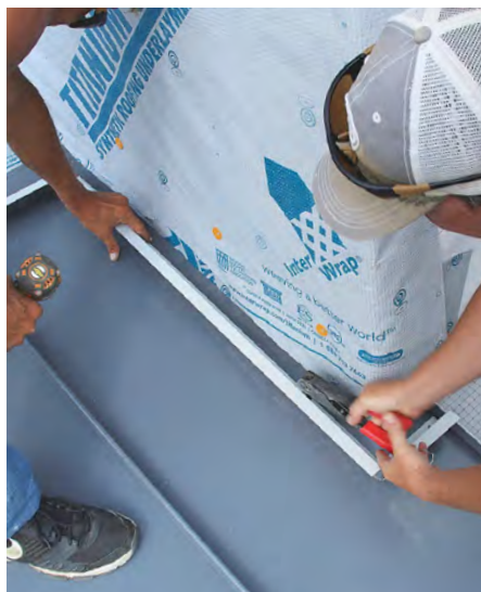
Rivets, not screws. Unnotched Z-strips connect to roof panels and sidewall flashing with rivets, but are not fastened down with screws, allowing movement.
