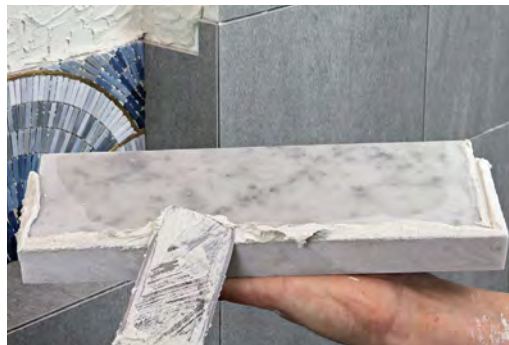
Butter the back edges. As always, to ensure a good bond, all mating surfaces get thinset.
