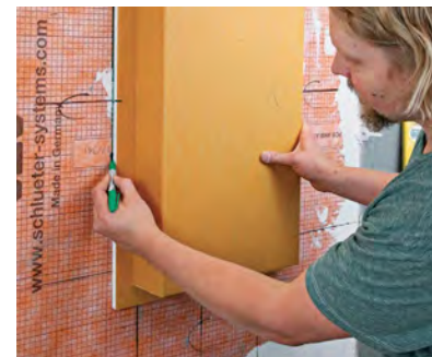
Flip and trace. The cutout has to include the flange on the front of the niche box, so flip it to trace the perimeter, using centerlines to aid in alignment.
