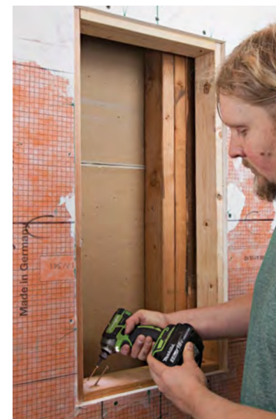
Add blocking. To simplify the box installation, toe-screw 2xs at the top and bottom of the opening, protruding into the opening.
