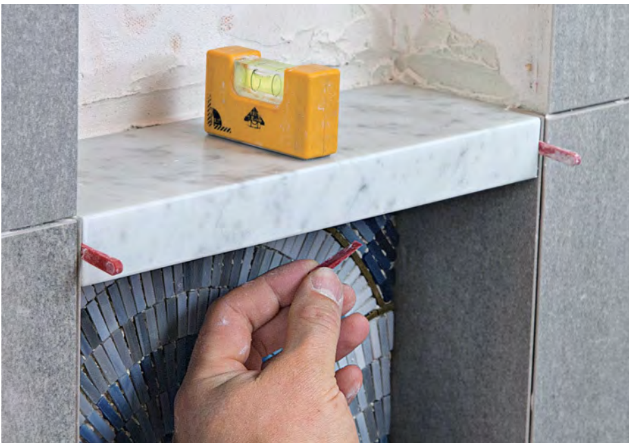
Slope it and gap it. The shelf needs the same subtle downward slope as the bottom of the niche, and wedge spacers ensure thin, even grout lines at the side and bottom edges.
