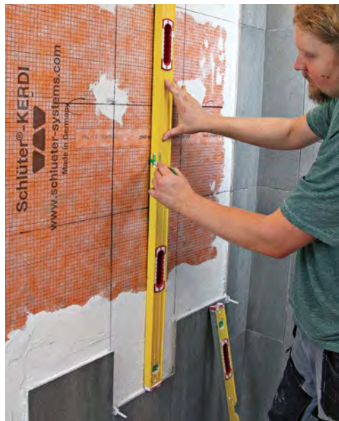
Extend the grout lines. After installing wall tile below and alongside the niche location, use a level to extend the vertical and horizontal grout lines to locate the cutout for the box.
