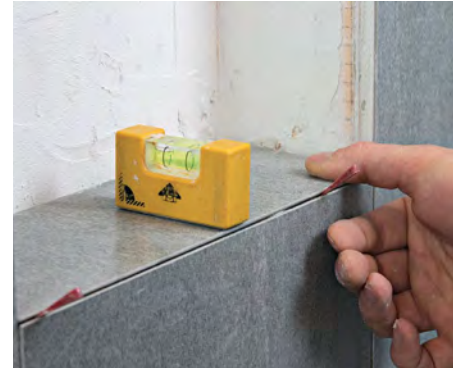
Pitch the bottom. Build up the thinset under the back edge of the bottom tile to establish a slope of roughly 1/16 in. over 3 in., just enough to offer drainage without the risk of shelf contents sliding off.
