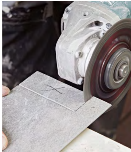
Notch the sides. Use a diamond cutting blade to create a notch in the side pieces that matches the thickness of the shelf but stops short of the full shelf depth.
