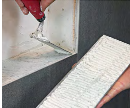
Back butter and scratch coat. All tile—wall and niche—gets thinset on its back side and a layer where it will sit to ensure a good bond.
