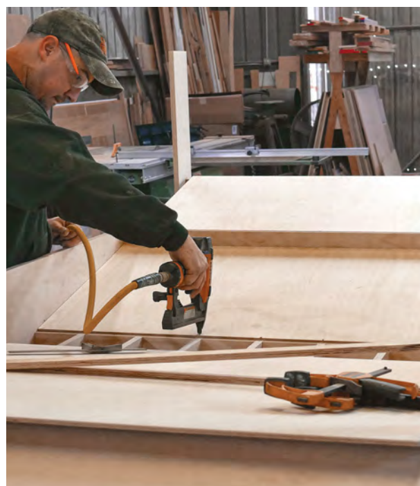
Install the legs and dust trays. Screw the legs to the apron and then attach the dust trays, made of 1/2-in. plywood, to the cleats. Finally, add 1/2-in.-tall strengthening ribs, made of 3/4-in. plywood, centered on the length of each tray and fastened with narrow-crown staples.
