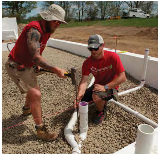
STEADY THE DRAINS
