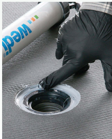
Attach the drain flange. Joint sealant goes below the flange, and a threaded collar pulls it tight. More sealant goes over the top.
