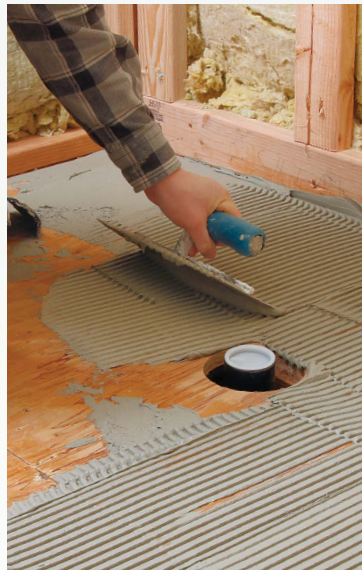
Apply thinset. Apply a notched coat of thinset mortar to the back of the pan and the subfloor.
