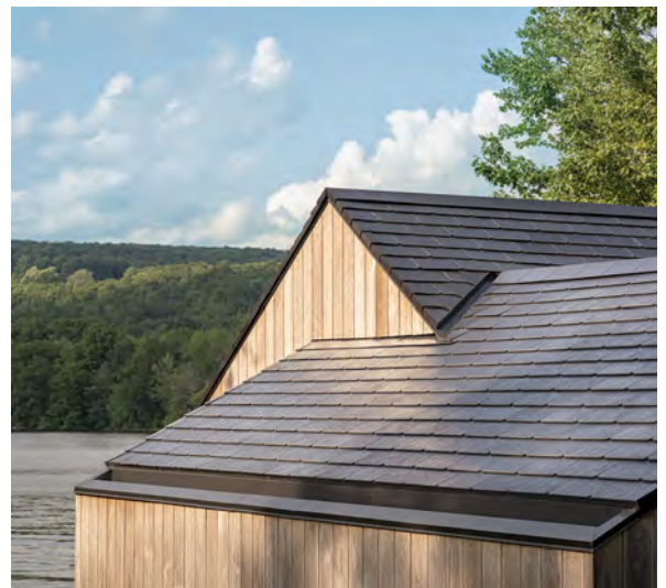
SOLAR-ENERGY SYSTEM Tesla solar tiles enabled more solar cells to fit on the small but complex roof shape than typical solar panels. Any energy surplus is stored in the Tesla Powerwall battery backup system in the garage.
